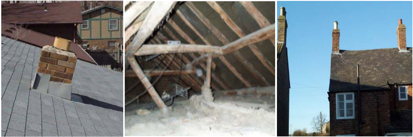
Figure 8 Some photos of defects that could occur in a roof space.
