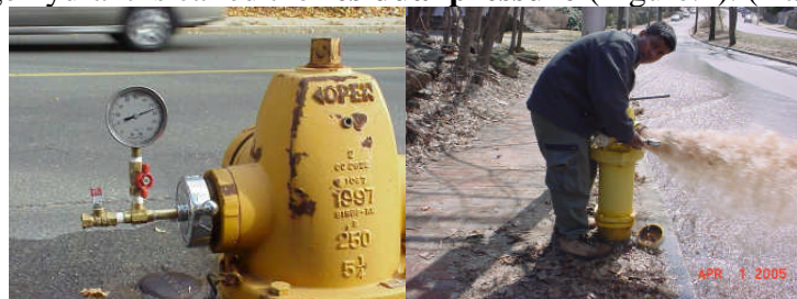
Figure 2: Gauge Hydrant and Flow Hydrant
