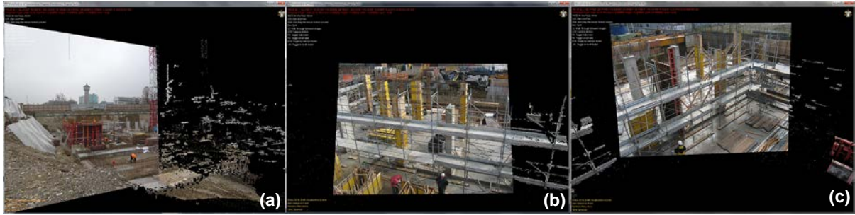
Figure 5: (a) Image-based 3D reconstruction of the building substructure with 30 4-megapixel images; (b) and (c) 3D point cloud models generated with 20 3-megapixel images highlighting the formwork and temporary scaffolding.
